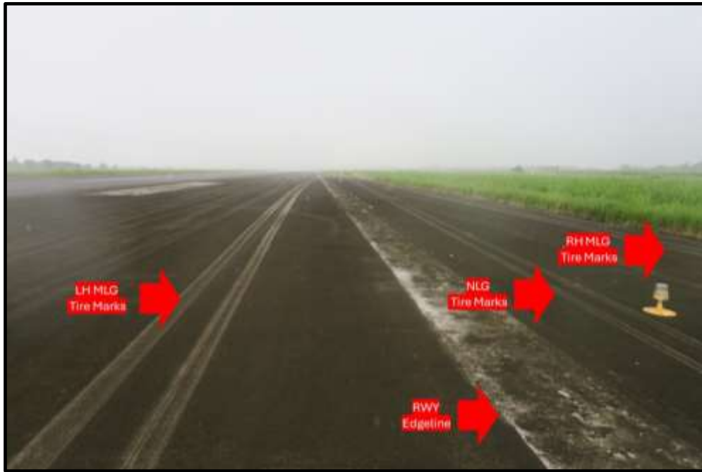
Figure 7 – Aircraft tire marks abeam the runway edgeline.
