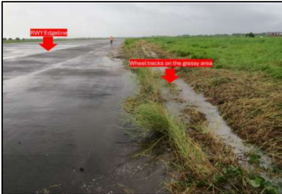
Figure 8 – Aircraft tire marks on the grassy area beside the runway.
