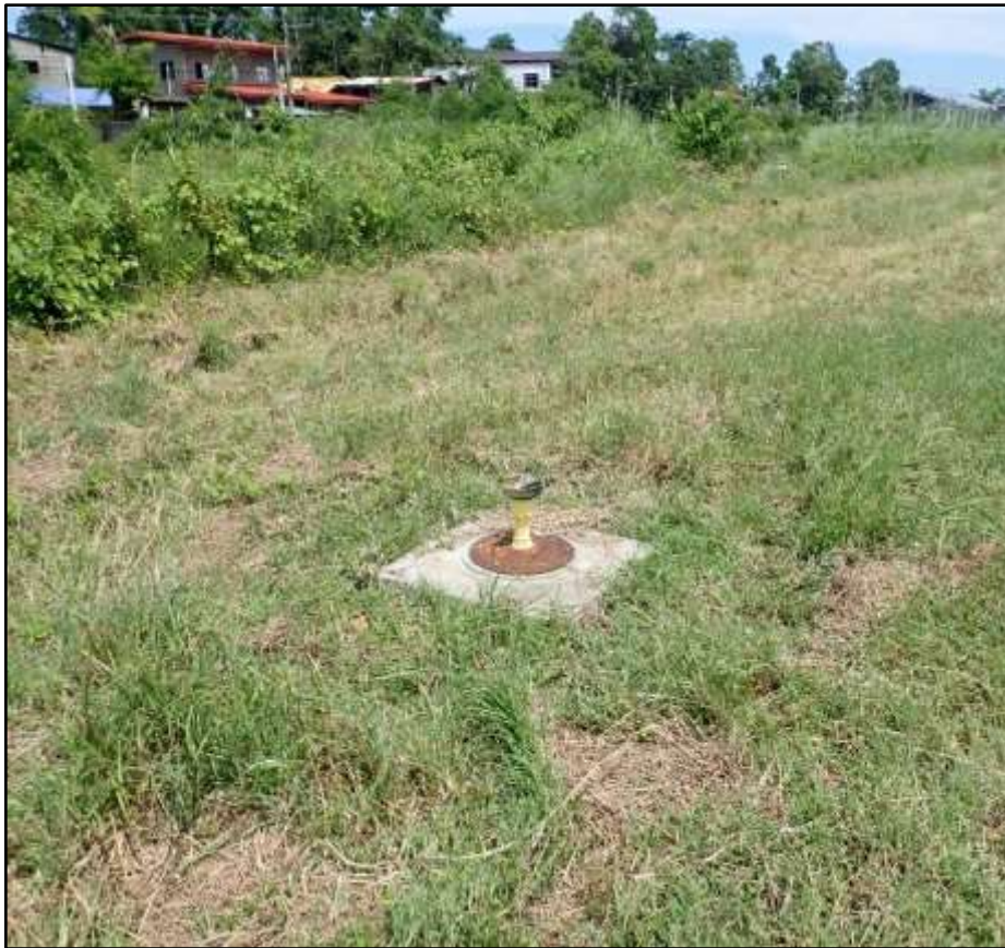
Figure 2 - runway side light.
