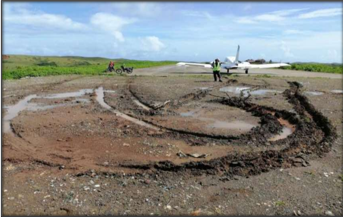
Figure 1 - RP-C4321 repositioned from the soft ground to the concrete pavement of the runway.
