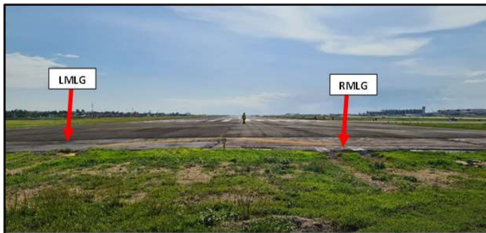
Figure 24 - The MLG visible tracks were seen before the pavement of RWY 22.
