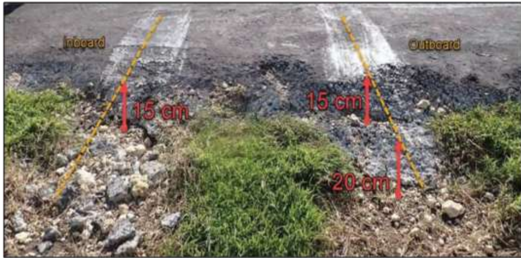
Figure 18 - The 15 centimeters step at of the cemented edge of RWY 22.
